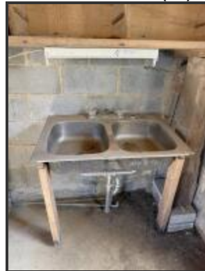
Basement sink (could work...just not hooked up at this time)
