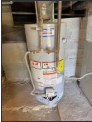
Hot water heater
