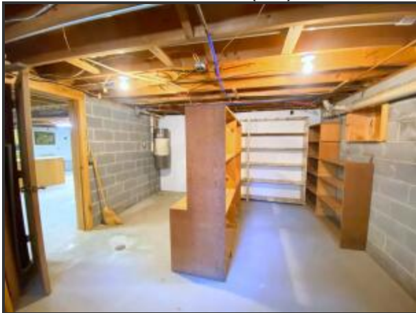
Lower level storage room with whole house vacuum (needs serviced)
