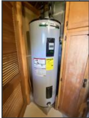
AO Smith hot water heater
