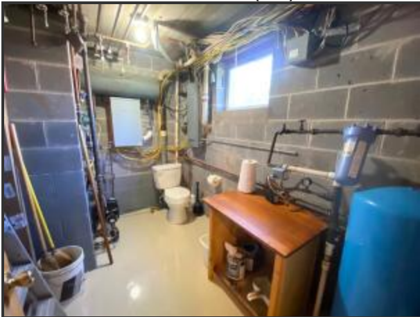
Lower level Mechanical Room &amp; half bath
