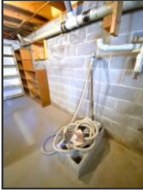
Lower level storage room whole house vacuum parts (needs serviced)
