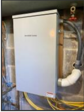
Briggs &amp; Stratton IntelliGEN Series generator panel
