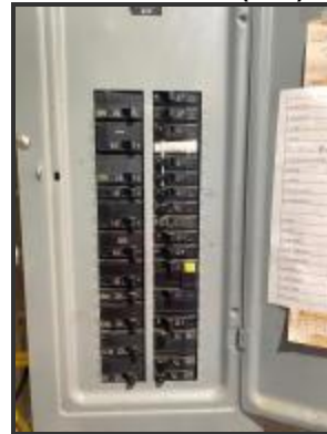
Lower level Mechanical Room - electrical panel
