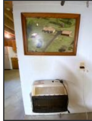
Lower level Recreation Room propane heater
