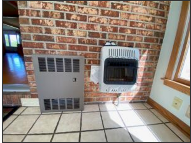
Sun Room propane heater (on right) and electric heater (on left)
