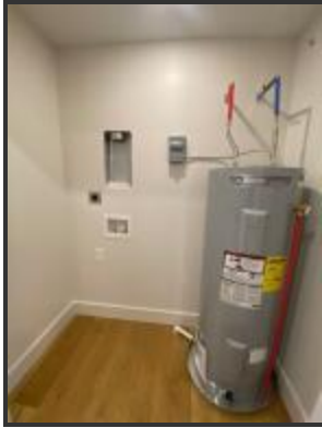
Utility closet with W/D hook-up
